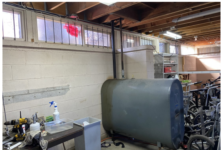
PHOTO 6: View of fuel-oil AST located in the basement of Site Building B.
