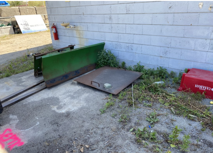
PHOTO 15: View of septic tank located adjacent to the west portion of Site Building C.
