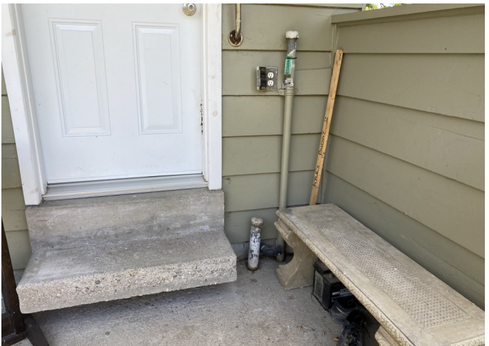
PHOTO 16: View of vent/fill pipes associated with a fuel oil AST at Site Building D.
