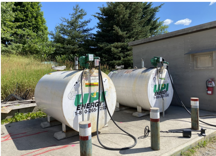
PHOTO 9: View of one (1) diesel and one (1) gasoline AST located adjacent to the east portion of Site Building C.
