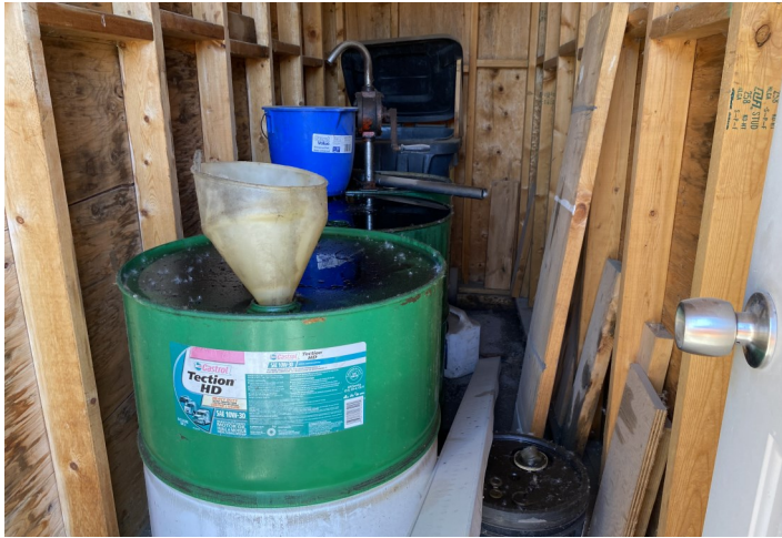
PHOTO 13: View of three (3) 205 L waste oil drums located 10 m east of Site Building C.
