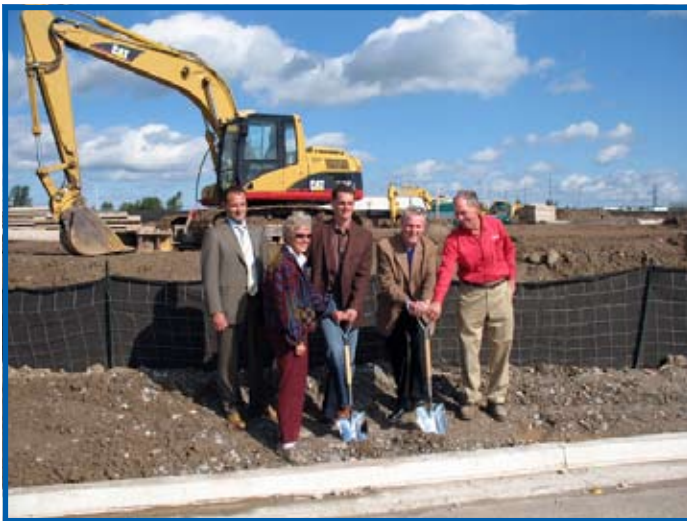
At the recent ground-breaking ceremony: (left to right) Marco Mancini, President, Urbacon Construction; Carol Chudleigh, co-founder, Chudleigh's Apple Farm; Dean Chudleigh, President, Chudleigh's Retail Bakery; Gordon Krantz, Mayor, Town of Milton; Tom Chudleigh, co-founder, Chudleigh's Apple Farm.
