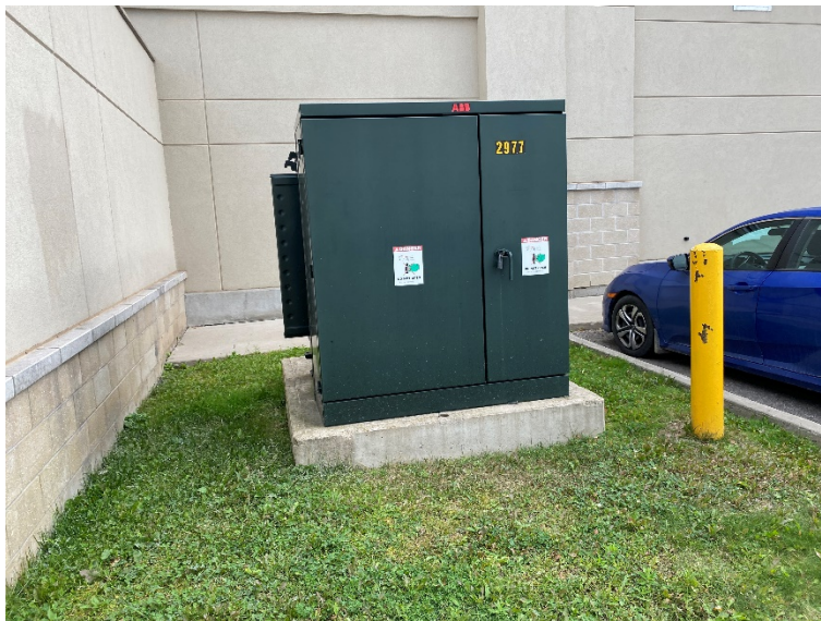
Photo 4 – General view of the pad mounted transformer located on the north side of 6941 Derry Road.
