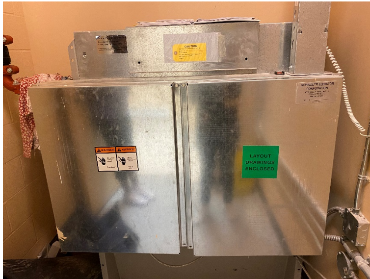
Photo 7 – View of the hydraulic oil reservoir associated with the elevator located in the building at 6941 Derry Road.
