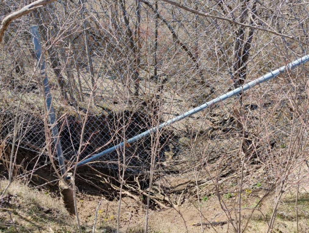
Photo 8: Slope failure in Cross-Section B-B area (looking southeast from top of slope)
