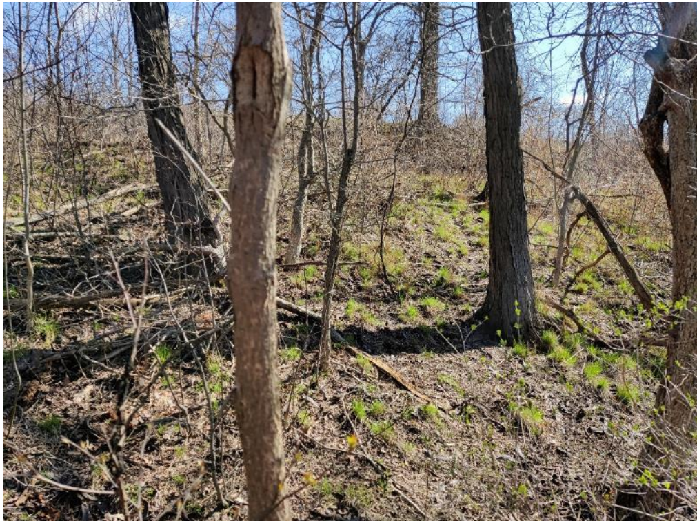
Photo 16: Slope conditions (looking north/upward from toe of slope at west of Cross-Section G-G)
