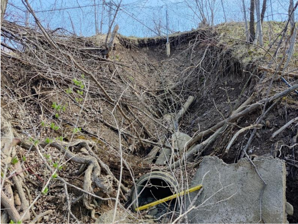
Photo 6: Erosion/Failure of Slope in Cross-Section B-B Area (looking north)
