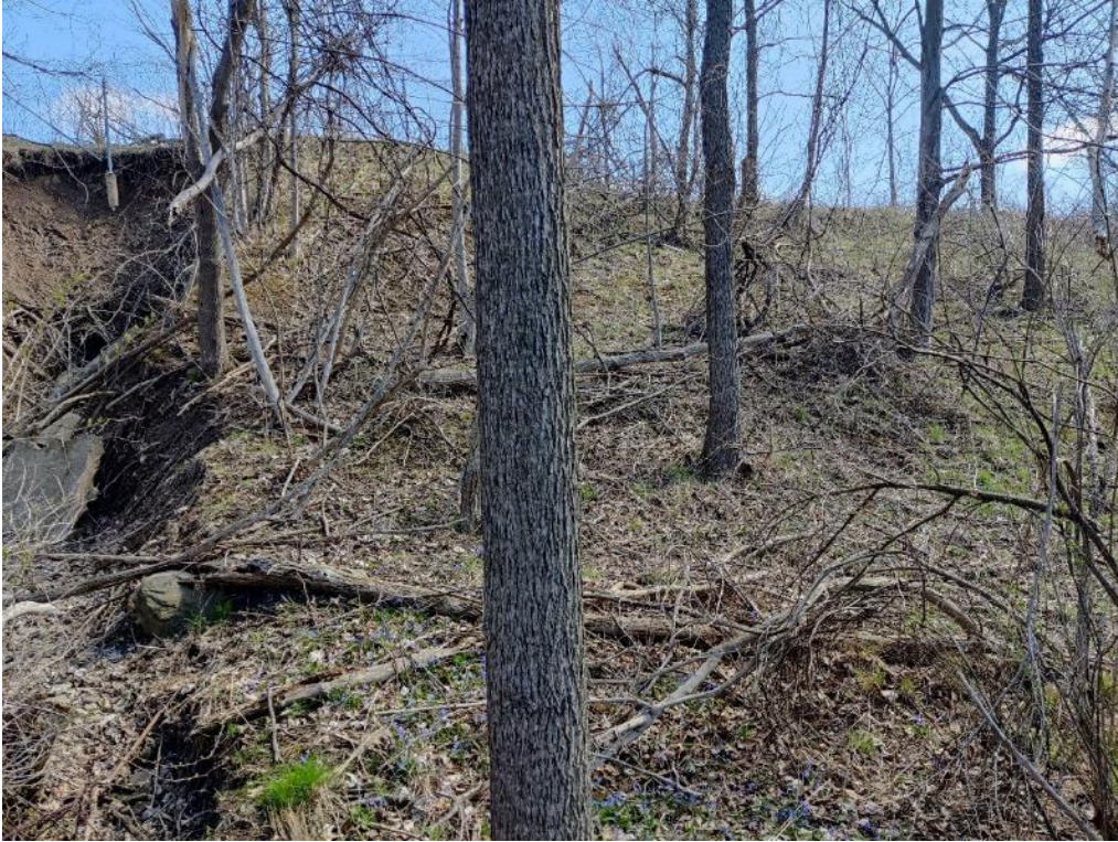
Photo 9: Slope conditions from Cross-Section C-C to Cross-Section D-D ( looking northeast from toe of slope)
