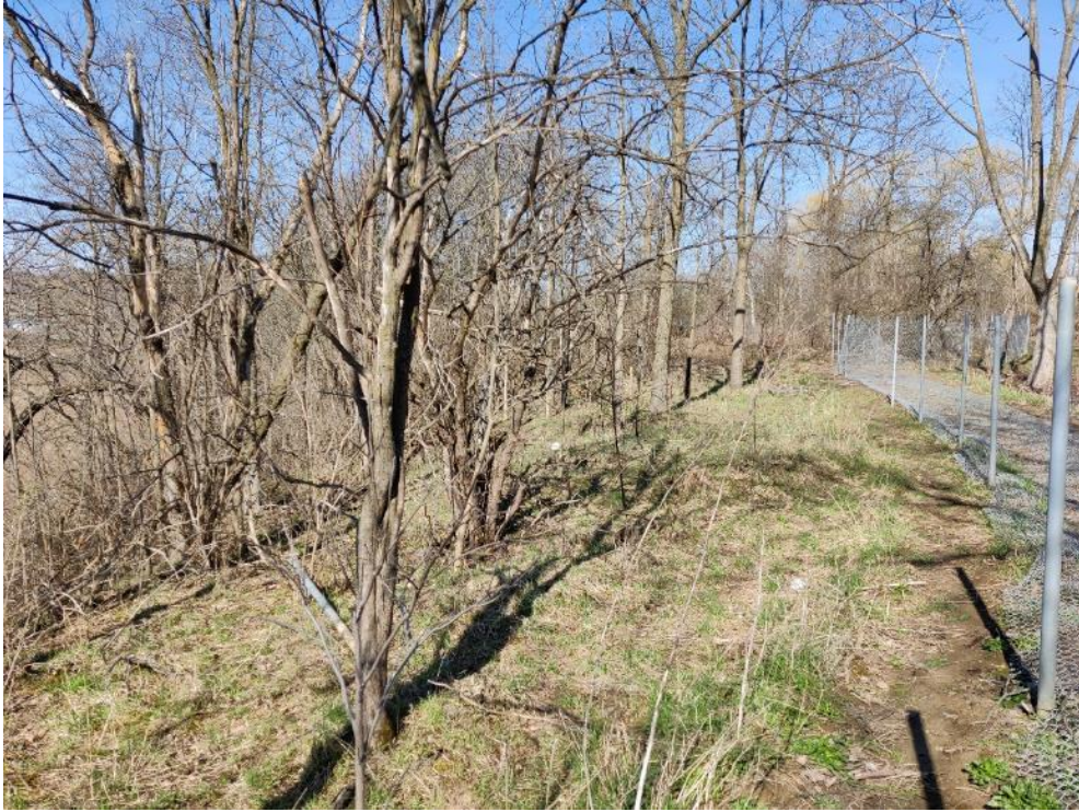
Photo 19: Top of slope conditions in area to east of Cross-Section I-I (looking west at top of slope)
