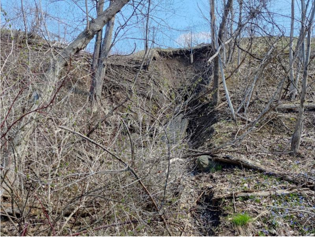
Photo 5: Slope conditions and erosion/failure in Cross-Section B-B area (looking north from toe of slope)
