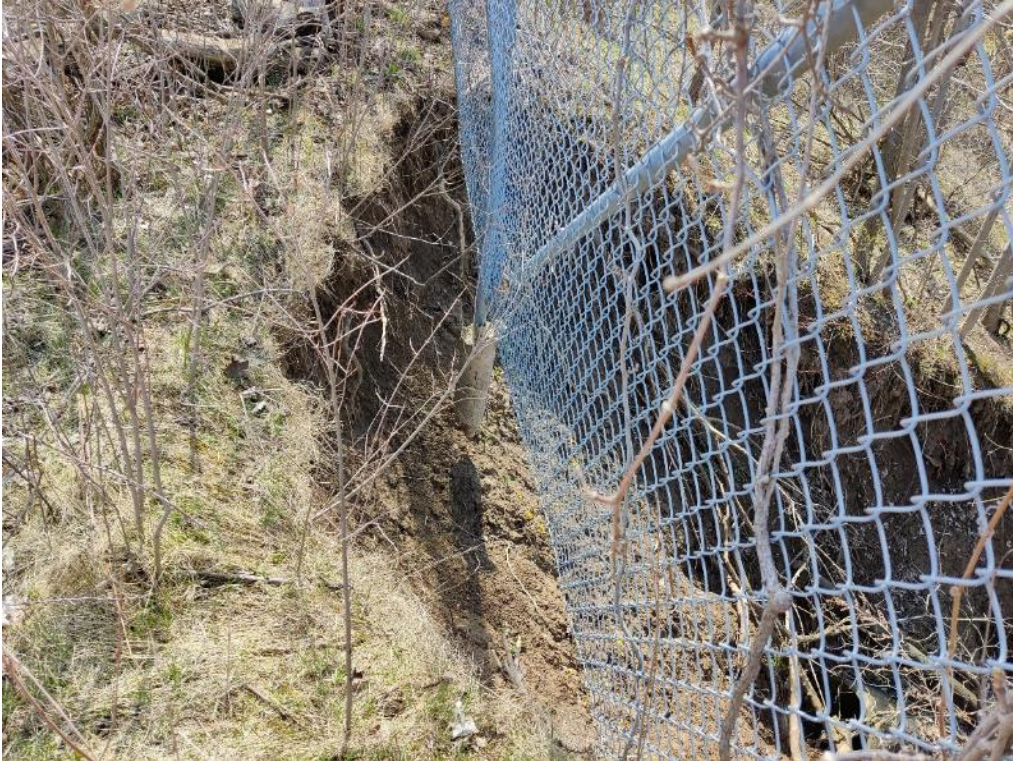
Photo 7: Slope failure at Cross-Section B-B (looking east at top of slope)
